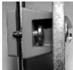
Lock-On Feature™ is inaccessible behind installed sign!
